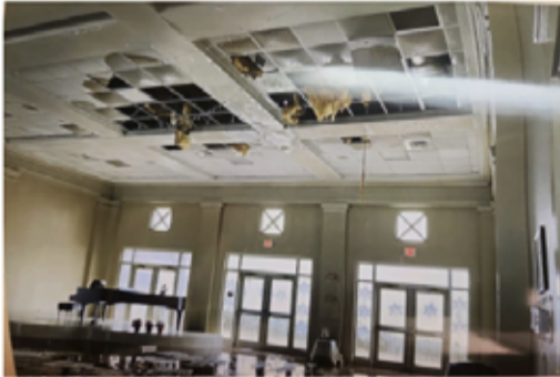
Pictured: Extreme cold weather in December 2022 caused a water pipe to burst at the Guntersville Senior Center, causing extensive damage. Plans are in place for renovations, with TARCOG assisting by securing grant funding for a portion of the project cost.
